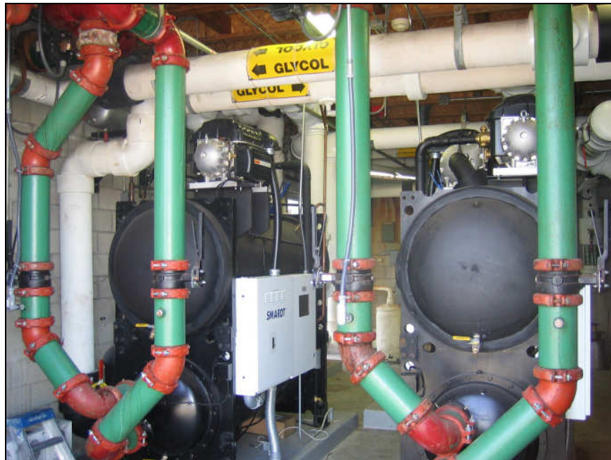
Figure 3: The two new 180-ton SMARTDT Turbocor chillers installed
