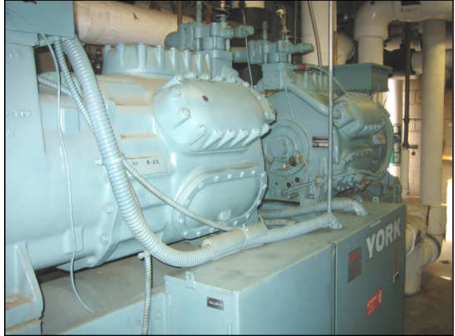
Figure 1: Pre-existing chillers, 165-ton, Manufactured 1991
